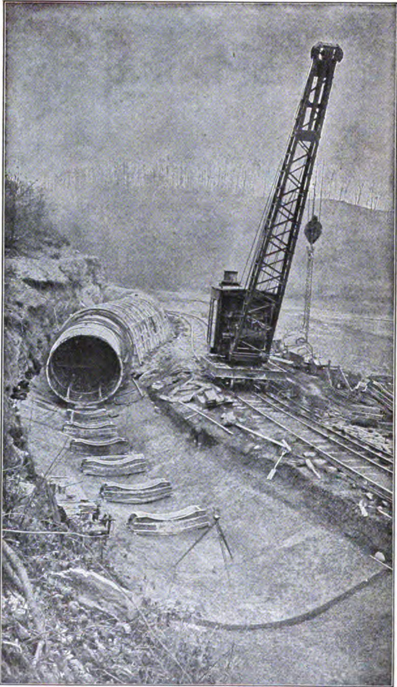
PLATE 176.—Contract 55. Reinforced Concrete By-pass Aqueduct. Shows successive stages of construction, concrete invert, pedestal blocks to support forms, etc.
